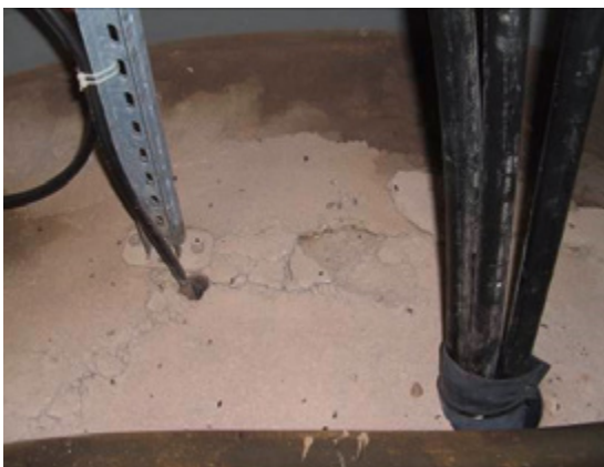
Figure 47: Cracks inside the tower; source: Gothaer, Edgar Sensen
