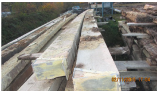
Figure 11: Beams deflection; source: VGH
