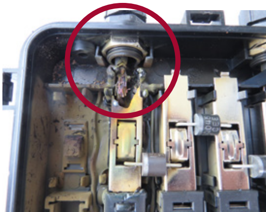
Figure 7: Electric arcs burned a cable and connector; source: PVGutachten.info
