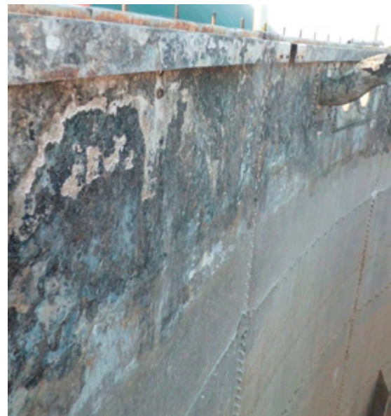
Figure 17: Corroded stainless steel wall after five years of operation. Damage costs: ~120,000 euros; source: DAS – IB GmbH
