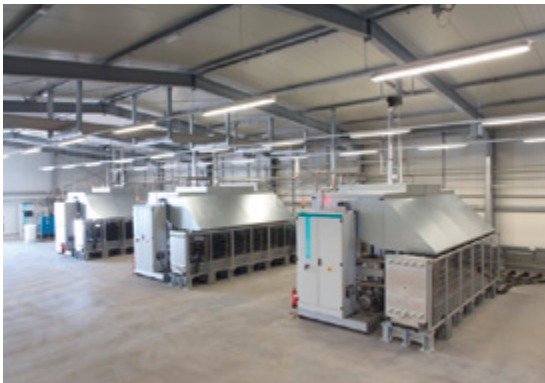
Figure 3: At the Energiepark in Mainz (Germany) an electrolysis system based on PEM cells is installed. The plant has a capacity of 1.5 MW and produces between 60 and 90 kg of hydrogen per hour. The electrolyzers are designed for a service life of 80,000 hours ( \hat{=} 10 years); source: Energiepark Mainz
