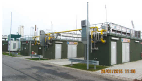
Figure 4: Pressure boosting station; source: VGH
