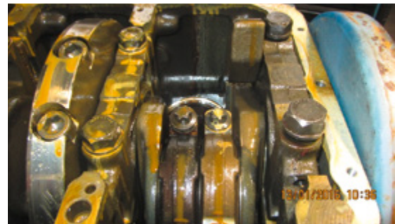
Figure 27: Coolant in lubricant oil, caused by damaged seals due to usage of the wrong coolant; source: VGH
