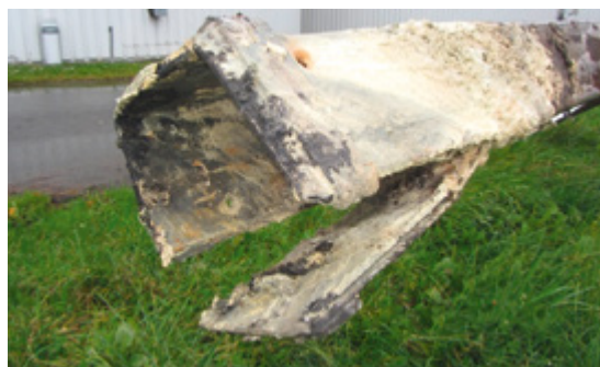
Figure 7: Breakage; source: VGH
