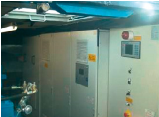
Figure 17: Converter cabinets, low-voltage power switches and control cabinet in a gondola; source: Allianz
