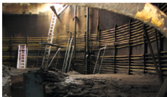
Figure 9: View into a tank with a surface-mounted heating system and high sediment layer. Near the upper image border, the remaining part of a large-blade agitator is visible. This tank had been in operation for seven years; source: VGH
