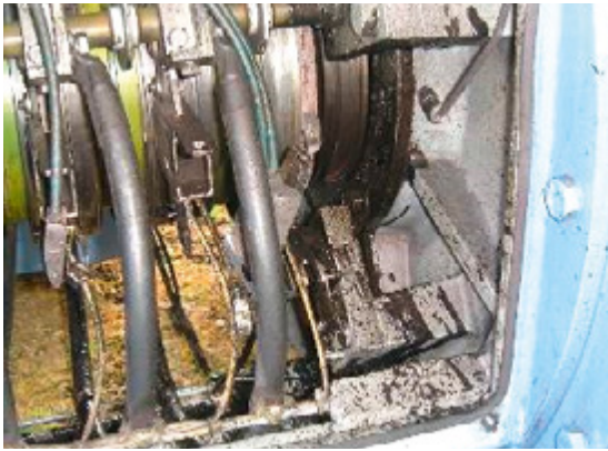
Figure 41: Slip ring housing of a generator contaminated with bearing grease; source: Allianz
