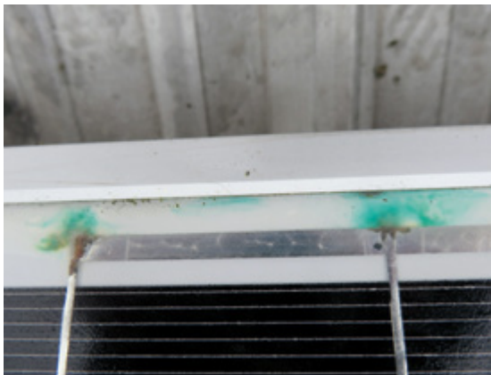
Figure 1: Corrosion of cell connectors due to humidity at the edges; source: PVGutachten.info
