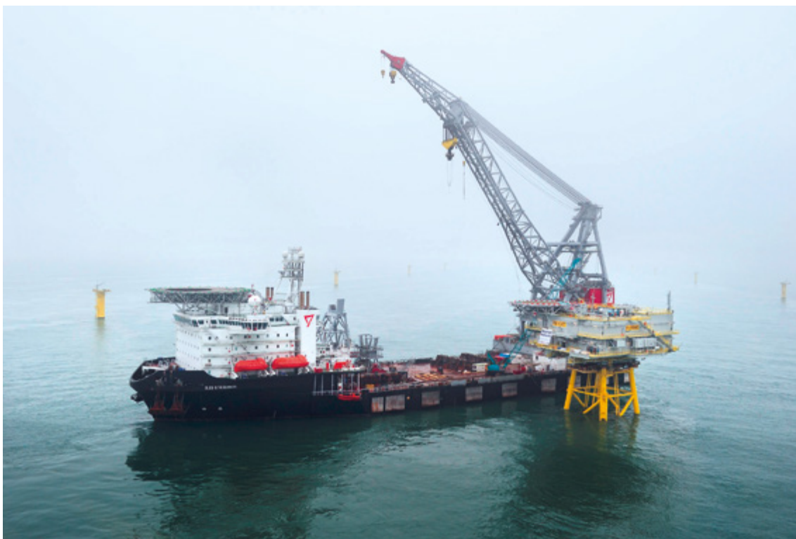
Figure 58: Transformer platform Riffgat; source: EWE
