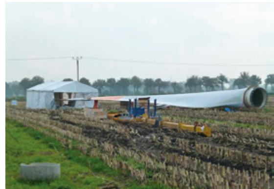
Figure 31: At low outdoor temperatures, repairs must be carried out in a heated tent; source: R+V
