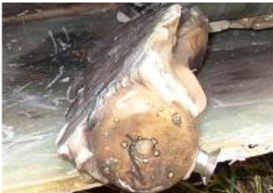
Figure 30: Receptor holders with receptors for the blades top and bottom shell. The holder is the connecting piece between grounding cable and receptors; source: Allianz
