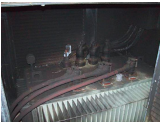
Figure 43: Fire damage on a 20 kV transformer due to lack of maintenance; source: R+V
