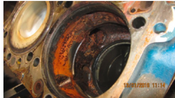
Figure 28: Excessive rusting all over the insides of the cooling circuit due to insufficient coolant treatment; source: VGH
