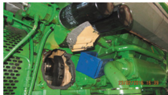
Figure 29: Despite warning messages the engine was restarted; source: VGH
