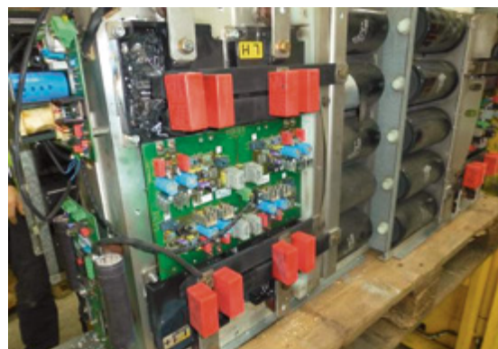
Figure 39: Inverter plug-in unit with defective IGBTs; source: R+V
