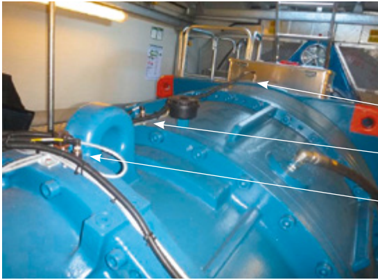
Figure 23: Sensors on the gearbox at the first planetary stage
