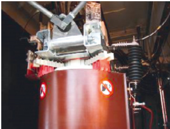
Figure 18: Side view of one of the three coils of a cast resin transformer in the gondola. In the upper middle part of the picture the attachment of the frame in the gondola is visible; source: Allianz
