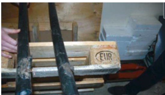
Figure 38: Internal wind park cabling damaged by dredging; source: Svst.-Büro Vogel, Ullrich Maug
