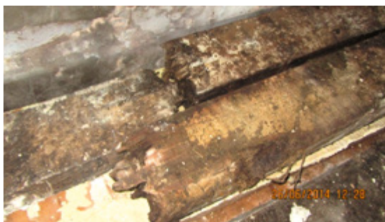
Figure 14: Corrosion; source: VGH
