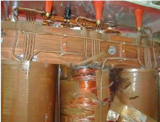
Figure 42: Transformer damage: Overvoltage from the power supply network with breakdown of the conductor insulation. The overvoltage protection was missing; source: Allianz
