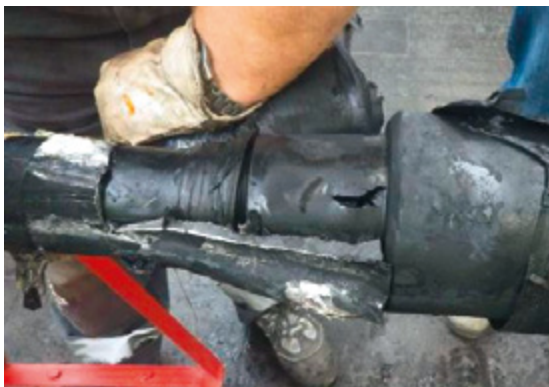
Figure 37: Failure of a 110 kV sleeve connection; source: 8.2 Group e. V., Nikolaus Kromm
